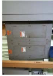
Electric Panel Strategic Replacements CMS, GLE, BEL, MBE, SMS
